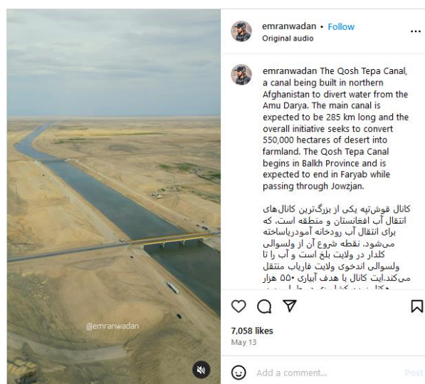
Figure 6: Kush Tupa Canal - being built in northern Afghanistan to divert water from the Amu Darya
